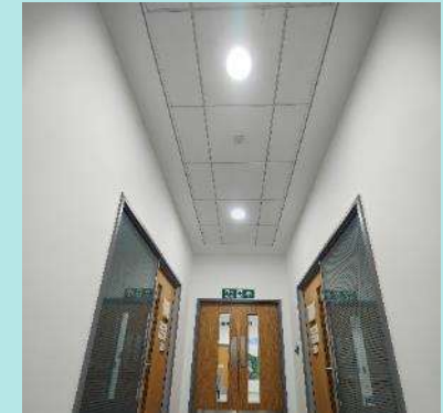
Newly installed LED downlights at Derriford
